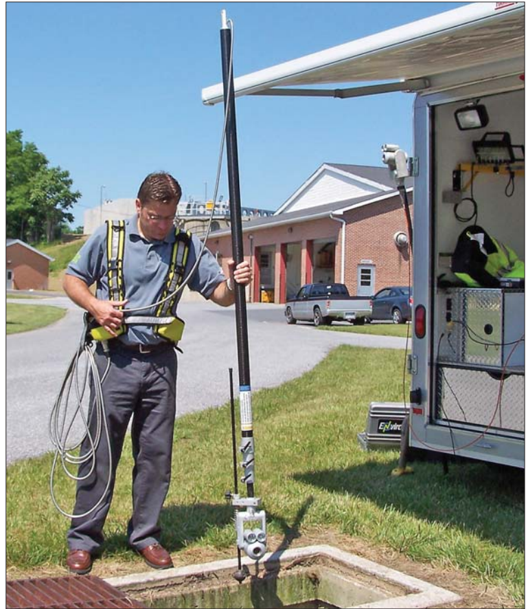
Kelvin Cherrington prepares to lower the QuickView system into a storm drain. The entire system — data and video recording equipment, battery pack, camera and pole — is seen in this view.
