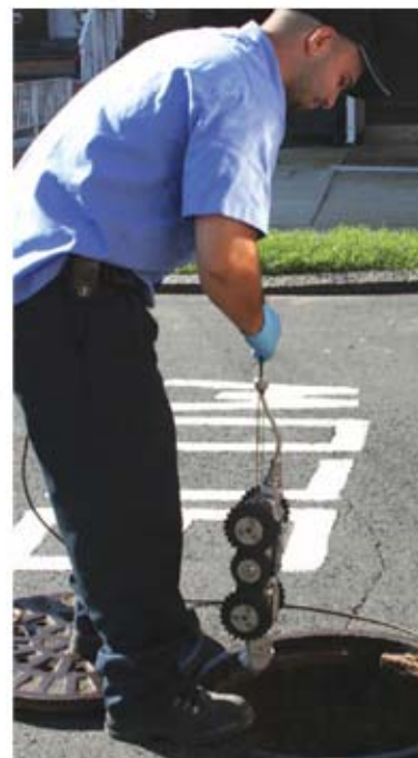
The sewer crew of North Bergen Township, N.J., upgraded their video-inspection equipment by adding a tilt/pan zoom camera, giving them even more flexibility and latitude. Photo: EnviroSight LLC
