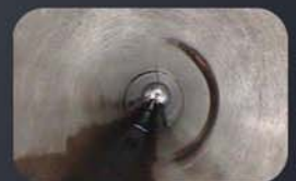
Sidewall & far illumination
